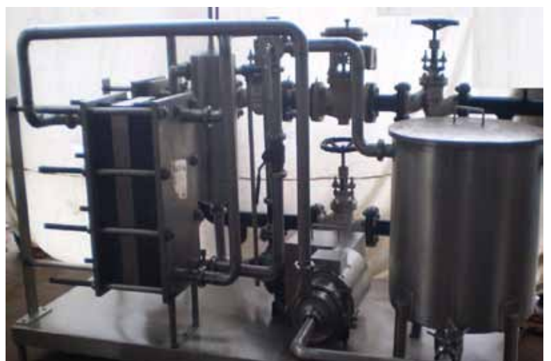
HOT WATER SYSTEM
